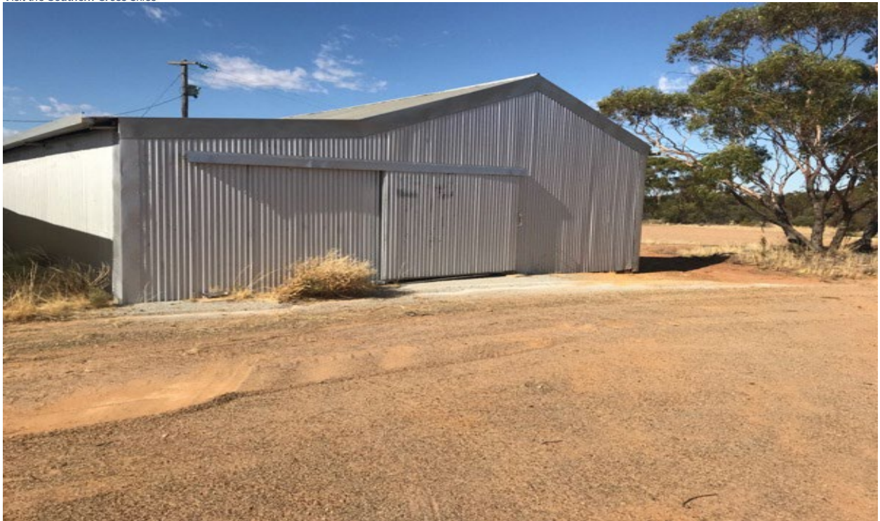
This is a steel framed, iron clad shed with concrete footings with a dirt floor.
